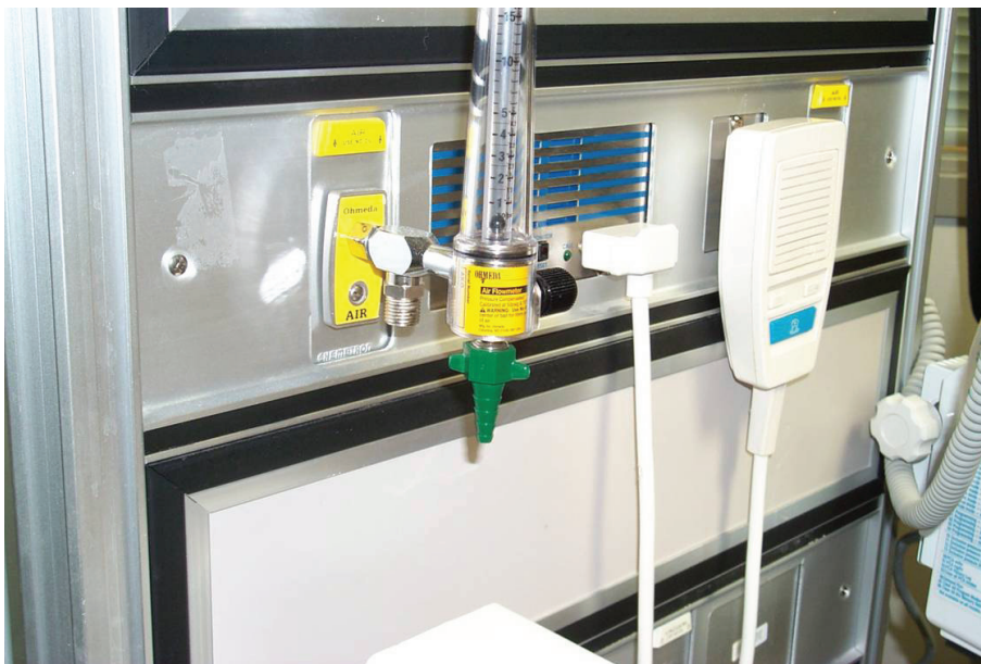
Figure 1. Device Hazard: Green Spigot
