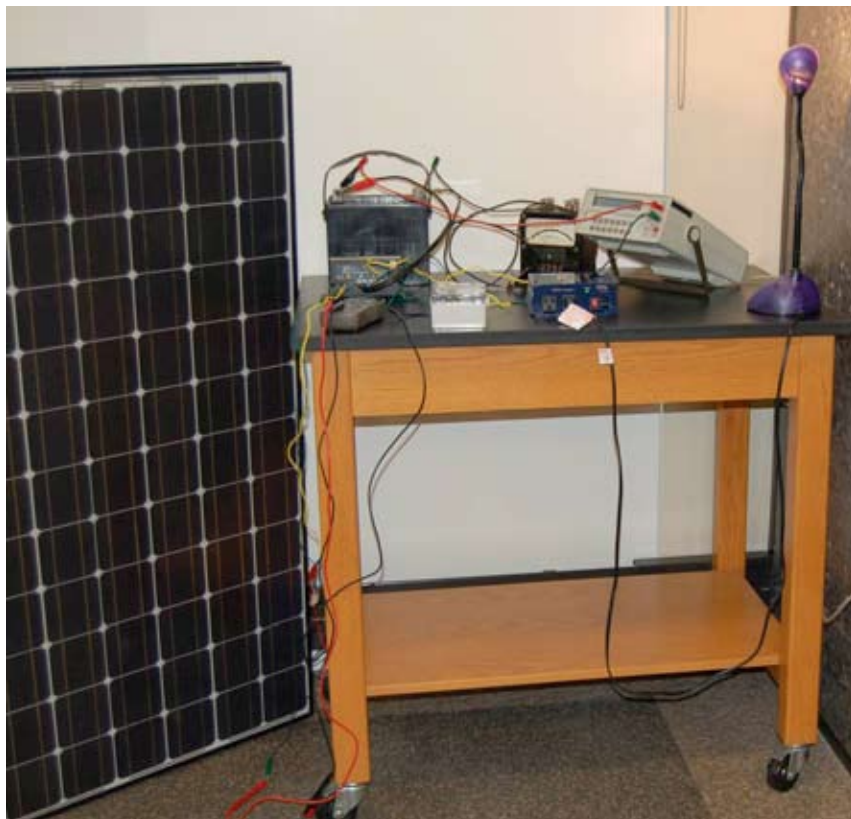
Figure 8. Components for a Transportable Photovoltaic System
